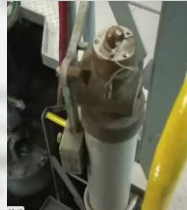
Sounding Pipe self closing
